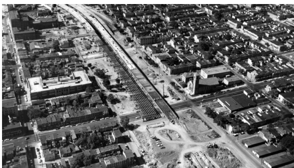
Highway construction in Wilmington, Delaware. Highways were also a tool of Urban Renewal, combining “slum clearance” with a connection to less crowded suburbs, with the added effect of clearing and bisecting “blighted” neighborhoods.
